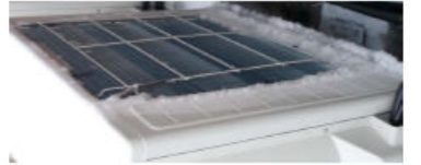
Frost on outside After defrosting
