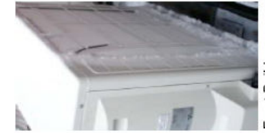
Frost Build up before defrosting
