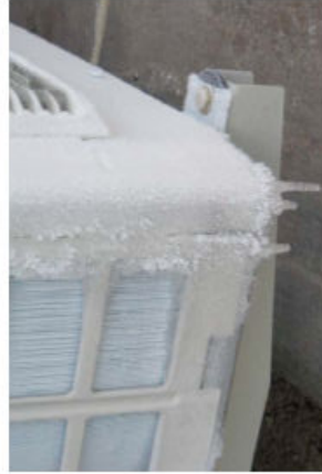
Frost Build up on the outside
